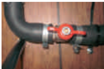
The fresh water tank's emptying valve in the open position
