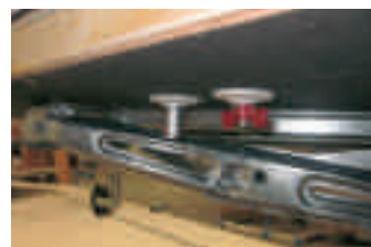
The grey water tank's external drainage valve
