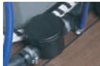
Water trap for the grey water tank
