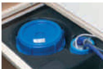
Fresh water tank
